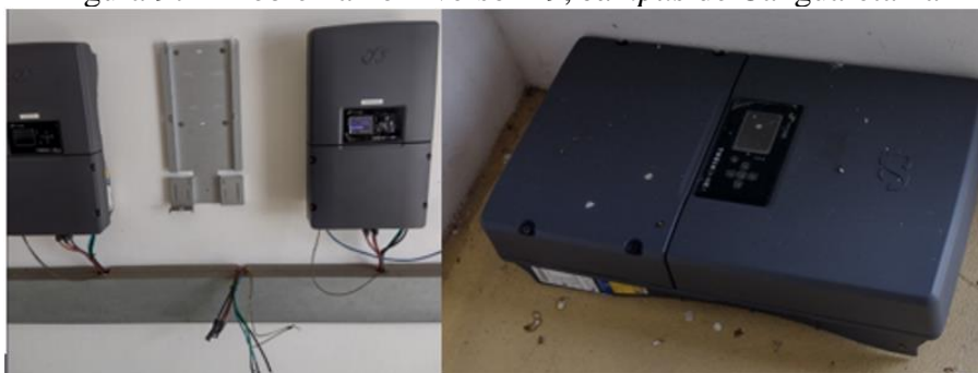
Figura 97 - Problema no inversor 19, campus de Canguaretama
